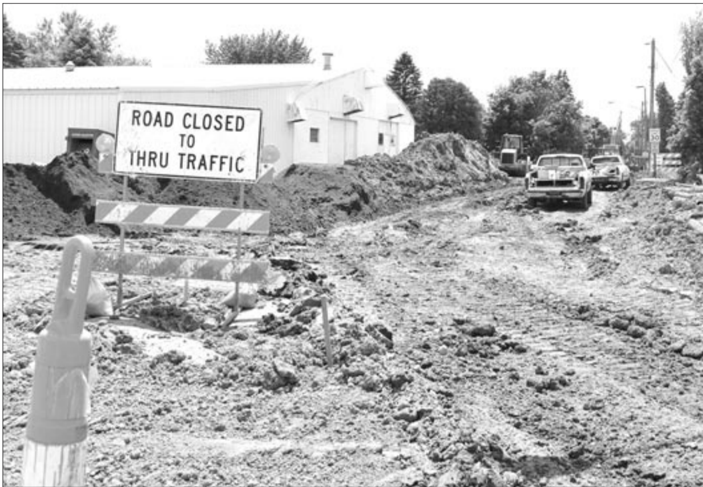
The reconstruction of Grove Avenue was a lengthy process in Silver Lake for the year 2013. Crews began work on the road beginning in May, and finished most
